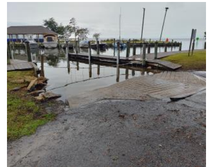
Debris at North Marina
